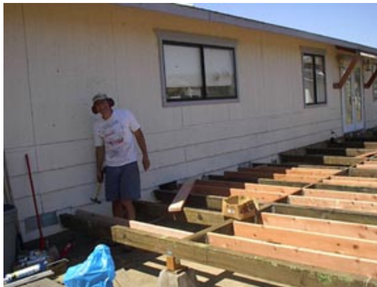
Robbie (Huh?) finishes up the deck framing; it's ready for the Trex decking crew!
